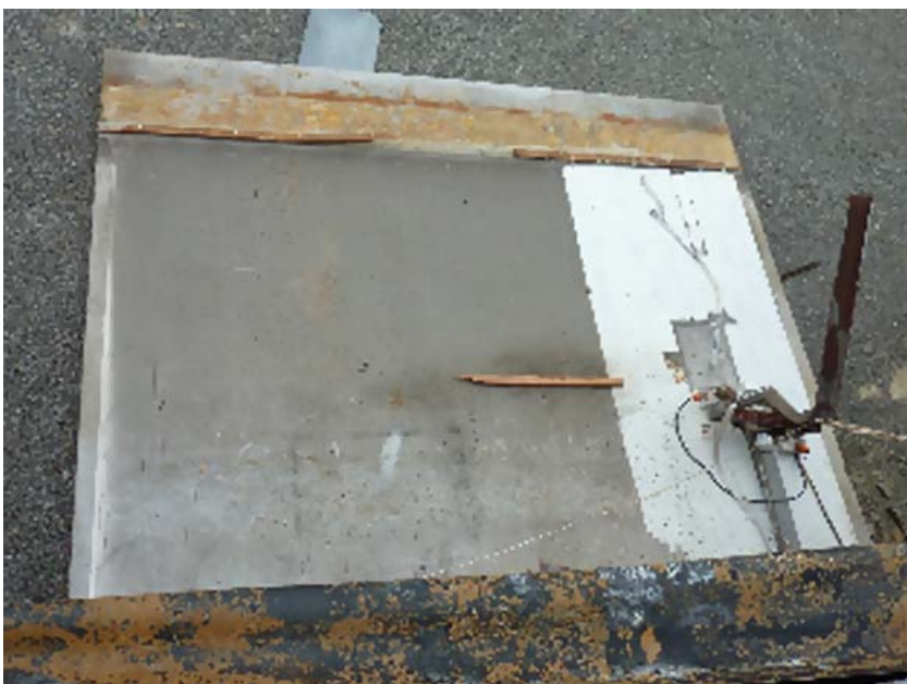
The fallen panel (which weighs about 10 tonnes) and the remains of the switchboard. What is left of the gutter can be seen in the foreground.
