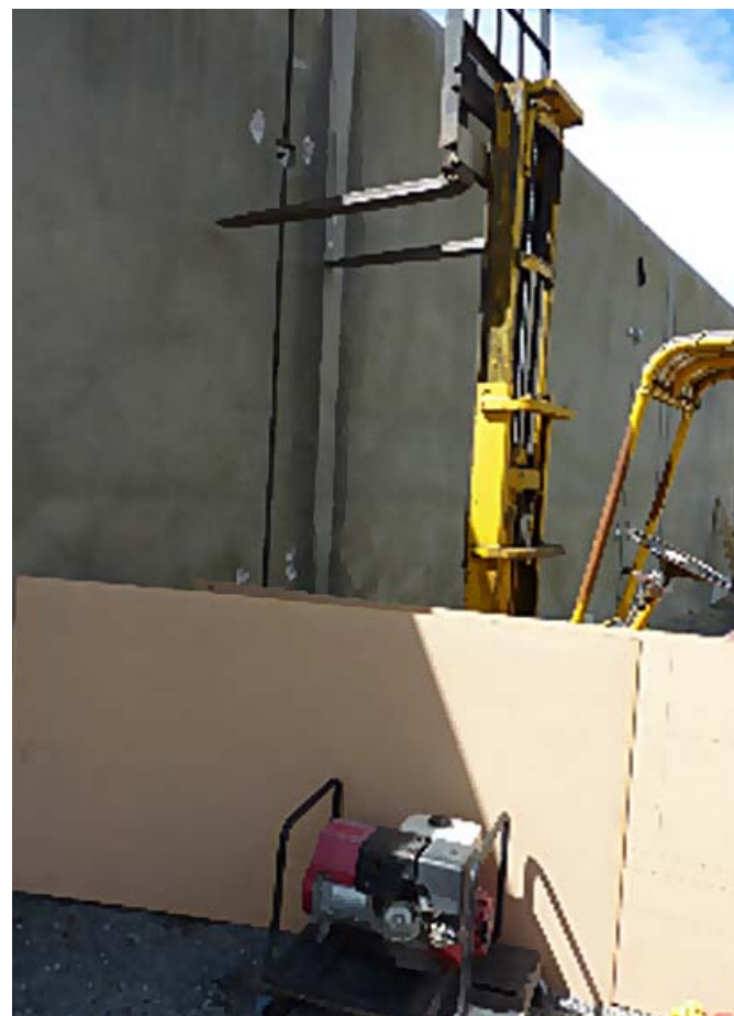
The forklift was moved along the wall, holding each panel as Fireworks Professionals’ staff drilled holes and put in the tie bolts.
