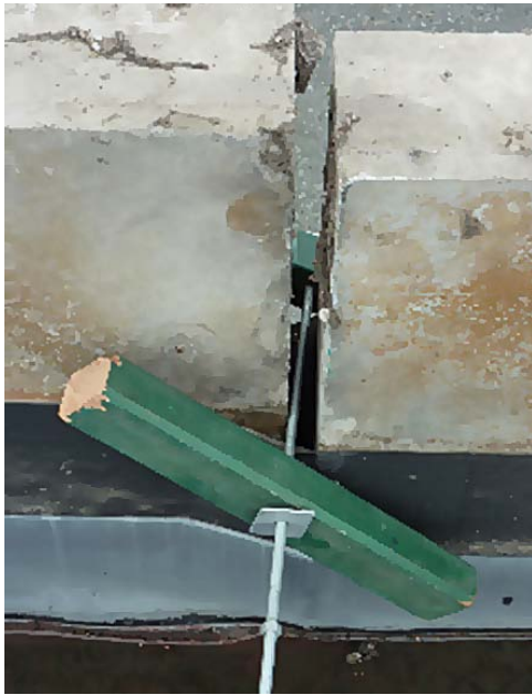
The attempt on the day of the earthquake to stabilise the remaining panels consisted of several of these locking the panels together, as not all the panels had shown signs of shifting.
